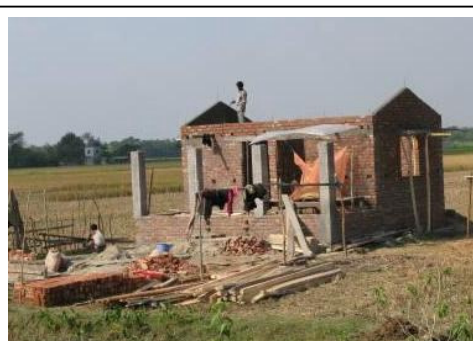
Building the final design – the beneficiaries manage the house construction while Muslim Aid supports with a series of cash grants and trainings.
