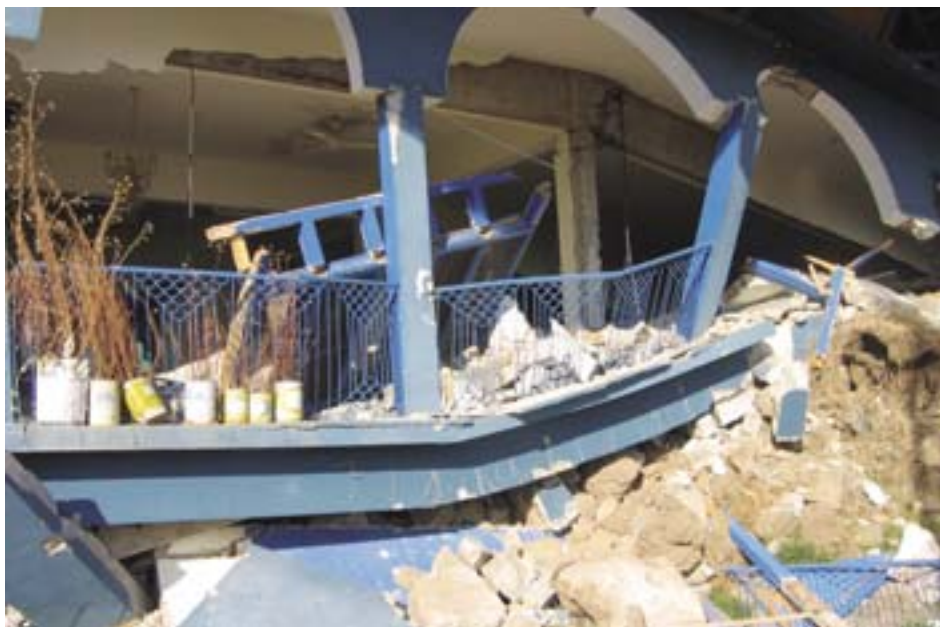
Partially collapsed house in Islamngar, Bagh District.
